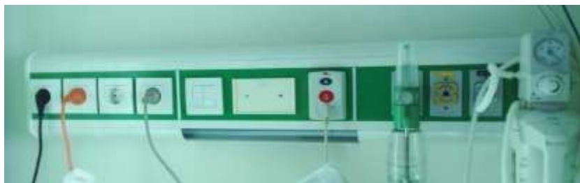
Figure 1. ICU RS Electrical Panel. Dr. Tadjuddin Chalid
